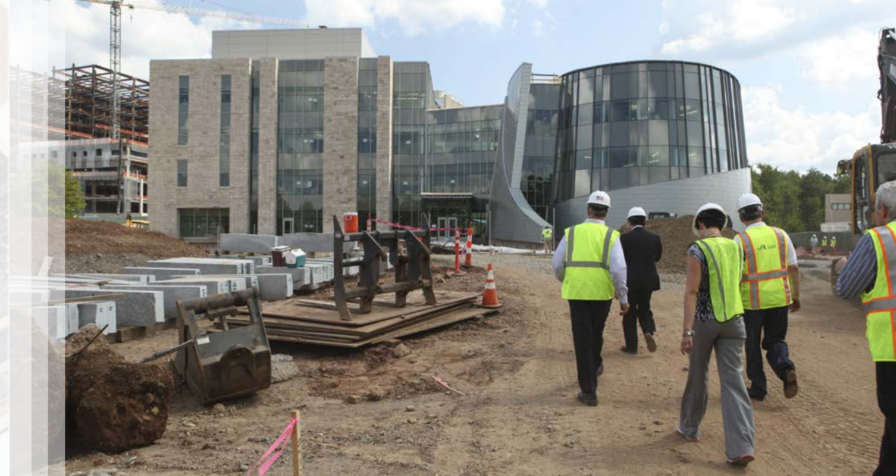
ABOVE Two months before the opening of JAX Genomic Medicine, staff members visit the construction site.
